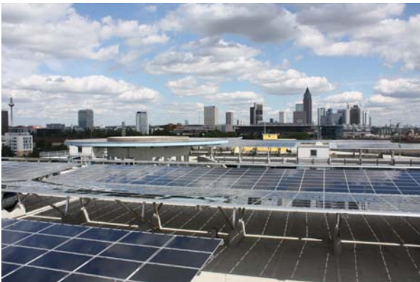
Picture 14: 0.8 MWp on a parking deck in Frankfurt
