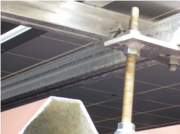
Figure 3: Corrosion signs in a coastal area
