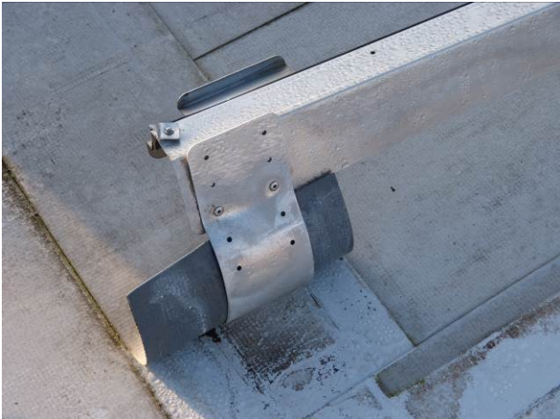
Figure 8 Extensive detachment of the glued lug
