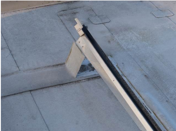
Figure 9 Failure by rupture of the glued lug
